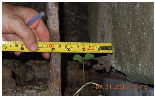
Transverse displacement of the Superstructure No. 5 over the Abutment No. 2. There is failure of the bolt, corrosion of the steel angle and evidence of water filtration.
