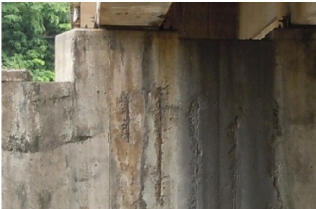
Damage on north side of Pier No. 1. There is no cover and therefore the rebar is exposed.
