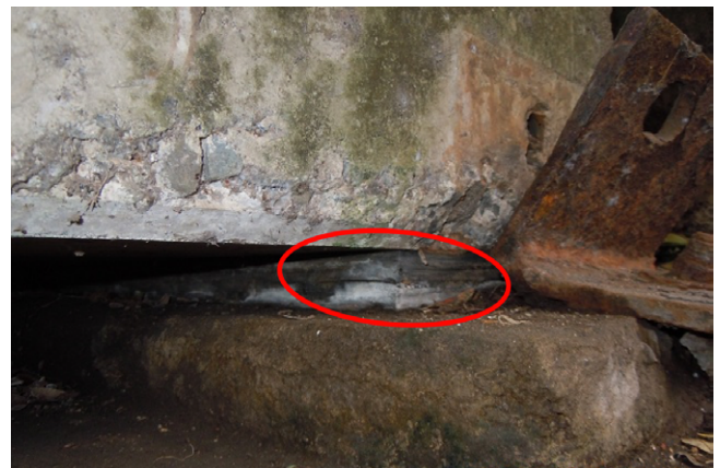
Crack on the neoprene pad on a bearing at Abutment No. 2
