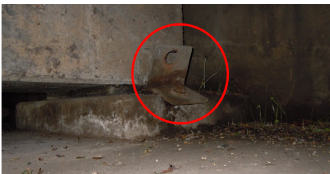
Damage on the bolts of a pedestal of Abutment No. 2, induced by the lateral force of the girders.
