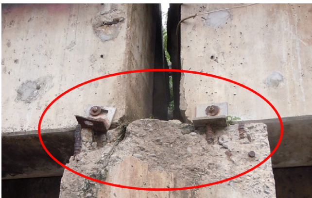
Damage on Pier No. 4. There is no connection between bolt and the bearing's steel angle, as well as cover detachment.
