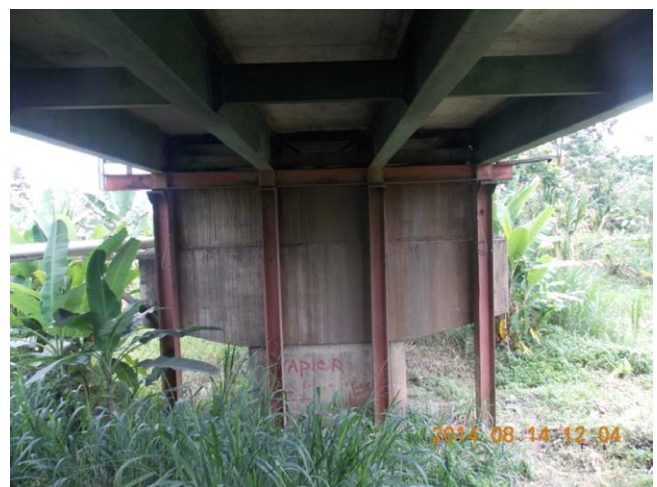
Metallic support structure built after the earthquake to prevent collapse of Superstructure 2.
