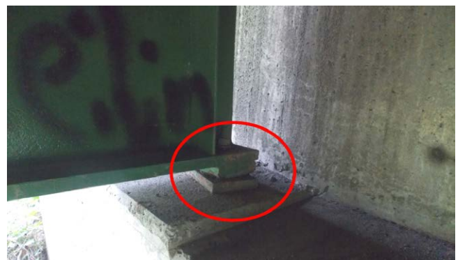
Displaced bearing on Abutment 2.
