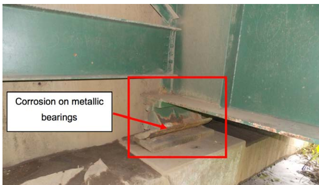
Rocking bearing tilted towards the headwall and corrosion found on Pier 1.
